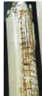
Deterioration of concrete due to improperly designed rebar splices and lack of reinforcement, often leads to premature splice failure.
